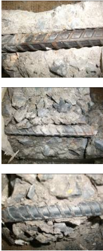
Figure 15. Exposed black deformed bar in mix 4 with 3 and 5cm cover (some rust).
