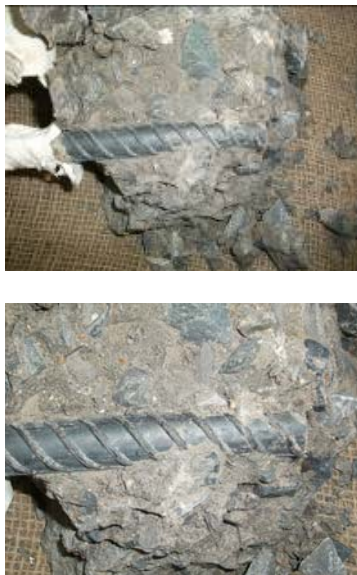
Figure 16. Representative exposed black deformed bar in mixes 1, 2 and 3 with 3 and 5 cm cover, (no rust).
